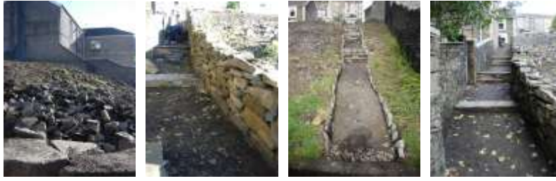
Katie Street, Blaengarw – disused land being prepared for community growing space, dry stone walling and footpath projects.
